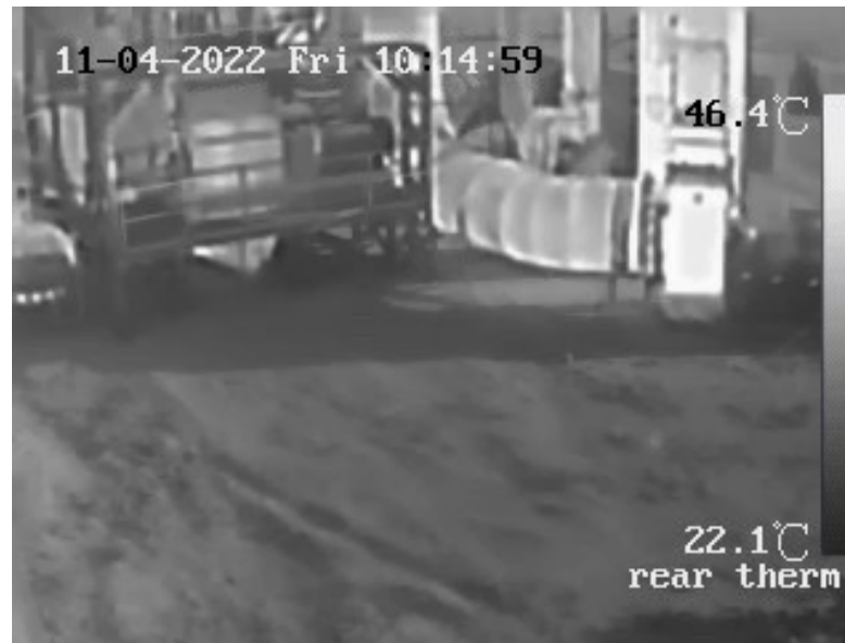
Thermal imaging camera photos (Courtesy of Shaw Renewables)
