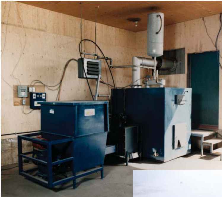
Power Line Pork, Borden, Prince Edward Island Facility Type: Pig farrowing farm System Size: 1 MMBH (two-boiler) Manufacturer: Grove Wood Heat Heating plant is housed in shed on left (lower photo). Fuel is delivered to overhead door and pushed onto shed's floor slab for storage, using tractor. Two side-by-side "Bioblast" systems (like the one in photo at left), located in the same shed, are sized at 45% and 55% of peak load. Each Bioblast consists of a tractor-loaded day bin (shown in foreground), a combustor (middle) and a boiler (rear).
